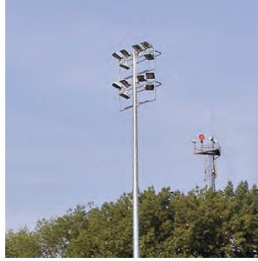
Fixed mast with ladder and twin platform
