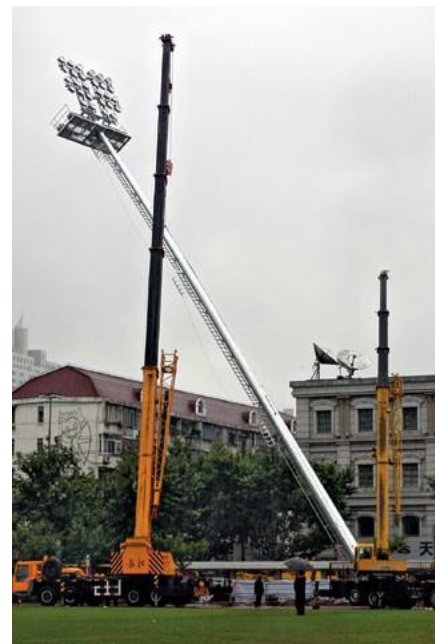
A 40m external-access mast example being lifted into position @ stadium with Mobile Crane.
