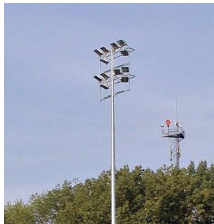
Fixed mast with ladder and twin platform
