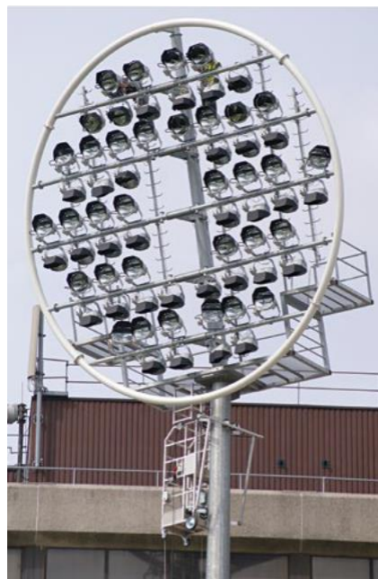
The manrider external-access system at work.
