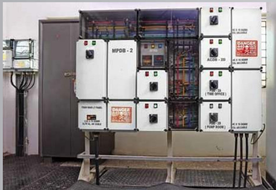
Distribution board at NPP Factory (6 October)
