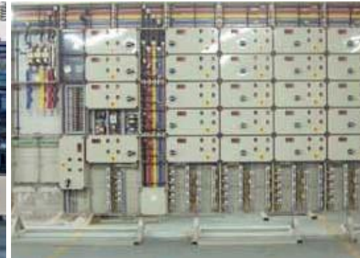
■ Motor control center installed in a large paper mill
