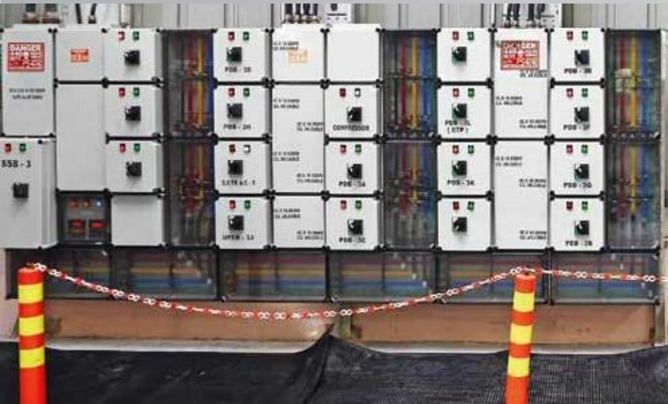
Power distribution boards installed at a light engineering industry
