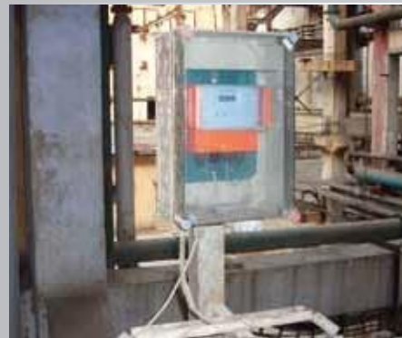
Control Cabinet at Venecia pump station
