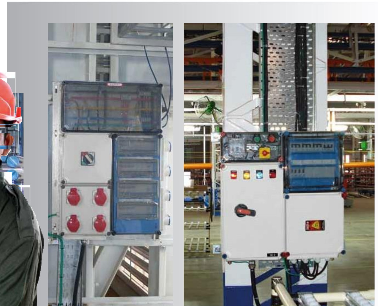
Shop floor distribution board with CEE sockets installed in an engineering fabrication plant.
