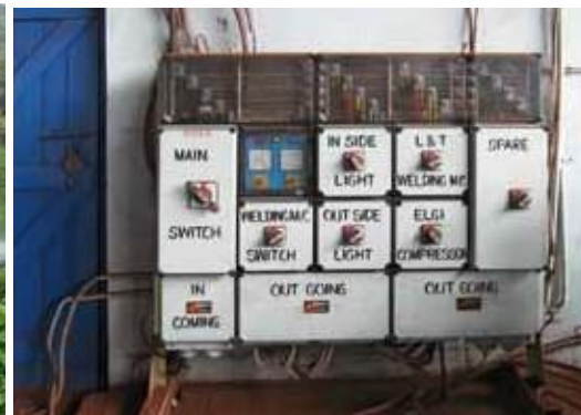
■ Power distribution board installed at a maintenance workshop of an iron ore mine
