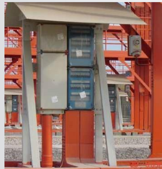
High mast lighting distribution board at ALEX Port, Titan Cement
