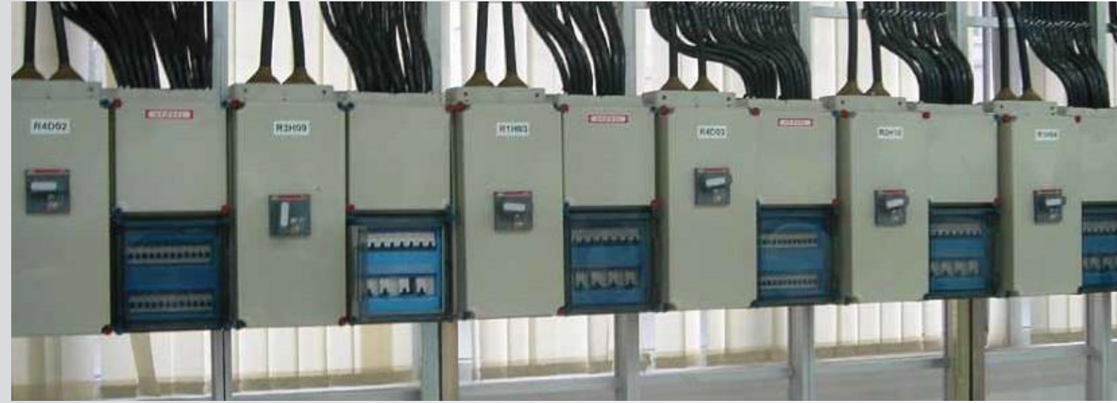
Lighting control distribution boards in use at a mobile phone manufacturing plant
