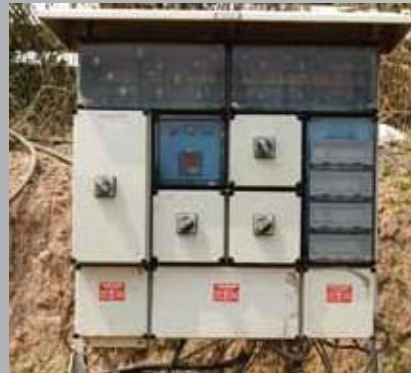
Sub distribution board installed at PICO GEN electric plant.
