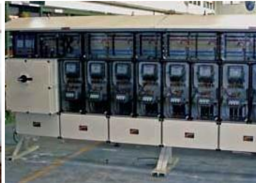
■ Metering panel with KWH meters for an electric supply utility company
