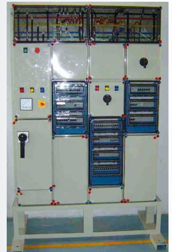
Main power distribution board for ESSO petrol station
