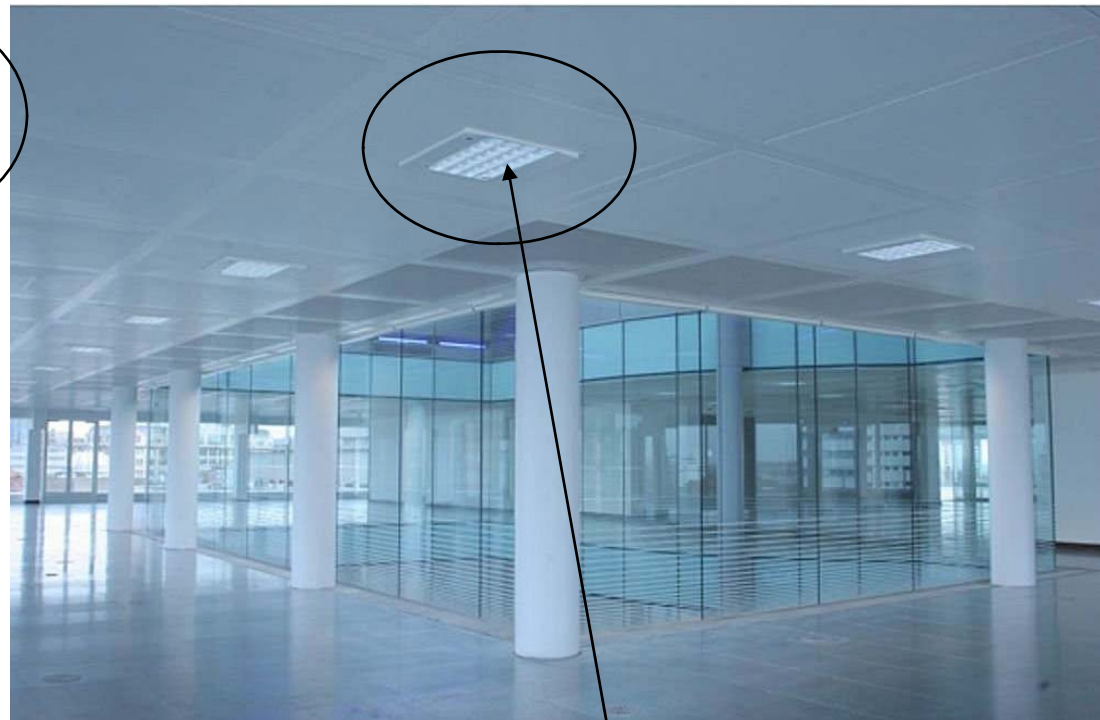
HVAC SYSTEM VENTILATION
