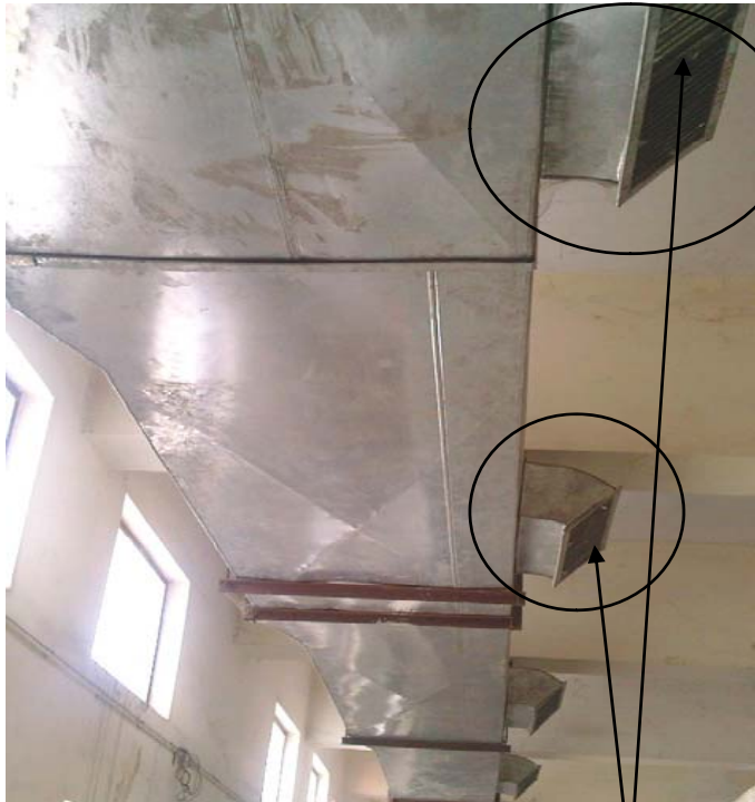
CENTRAL AC VENTILATION TO THROW COOLED AIR
