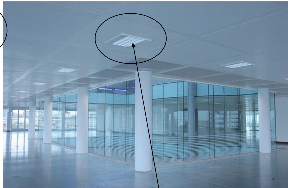
HVAC SYSTEM VENTILATION
